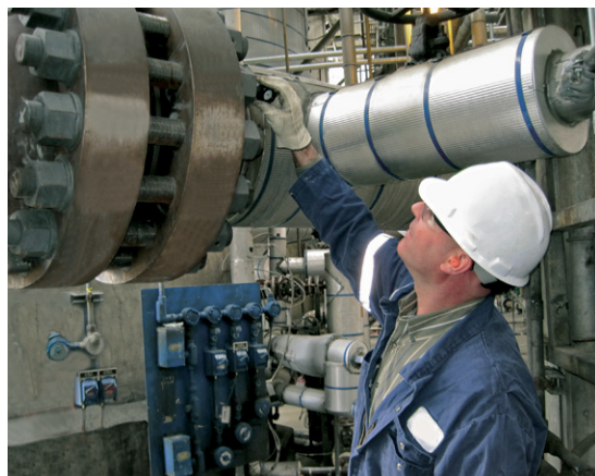
Reading bolt load on SPC4™ bolt with gauge
